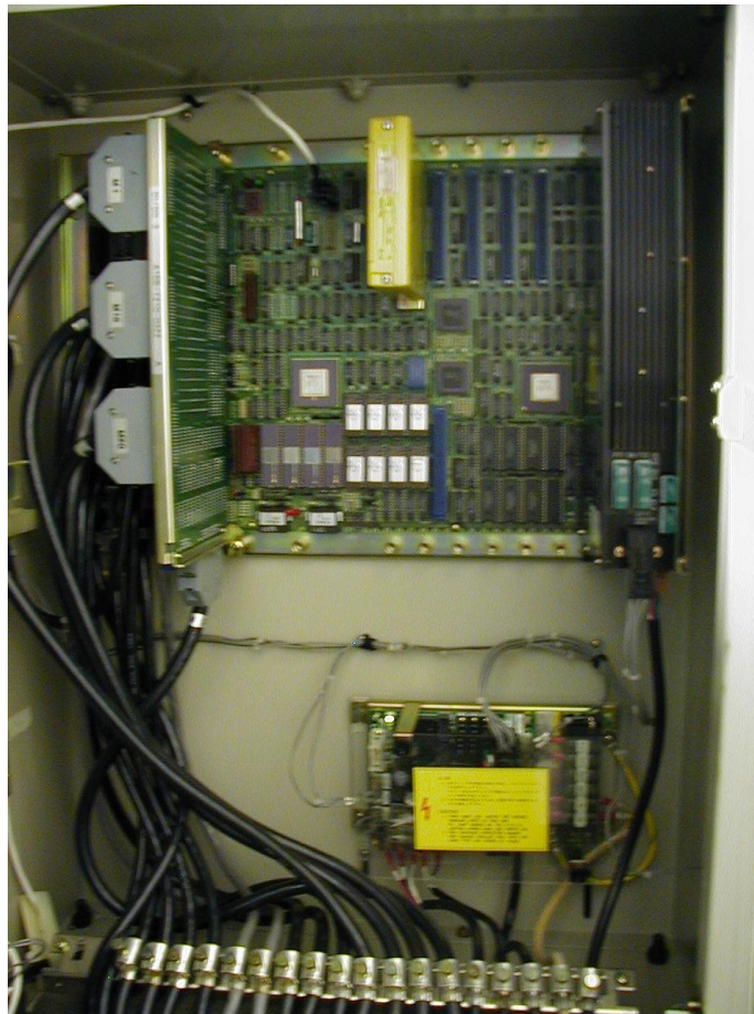
Fanuc 10A – all upgraded (no empty sockets)
